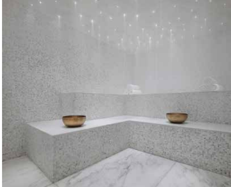
A flat ceiling in a steam room can work perfectly well as long as it is correctly designed, insulated and finished.
