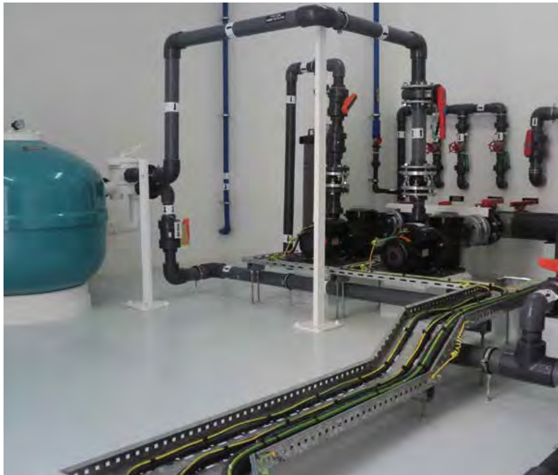
Example of a small plant room for maintaining a hot tub or spa pool.
